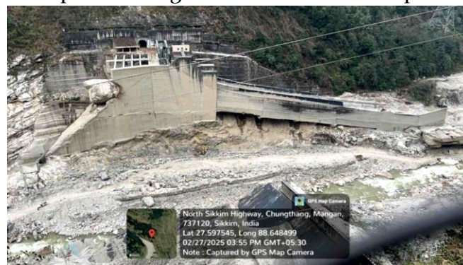
The 2023 GLOF Damaged Teesta Stage III Dam at Chungthang
