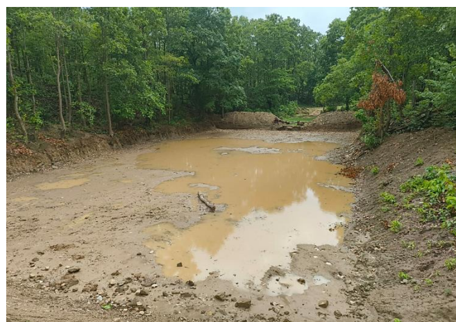
Earthen Check Dam & its poor Water Storage Capacity
